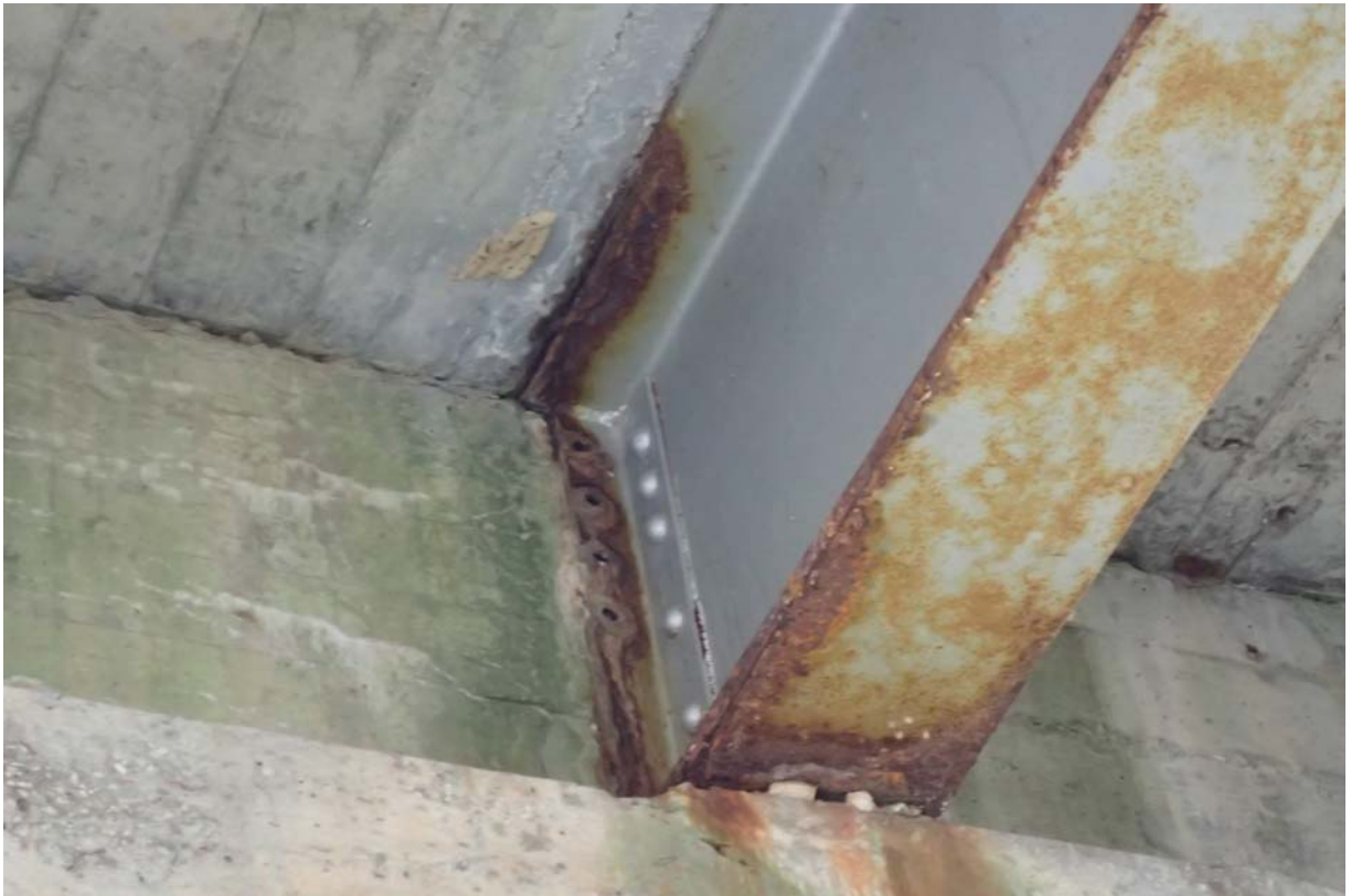
Typical view of beam 3 from upstream at abutment 1 (downstream face). Notice the moderate rust/corrosion of the web and flanges.
