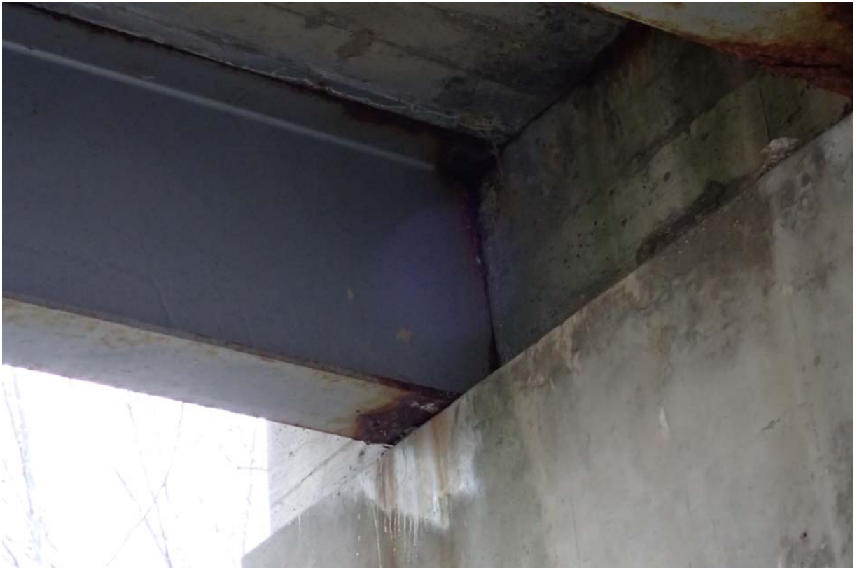
Typical view of the upstream beam at abutment 2. Notice the moderate rust/corrosion of the web and flanges.
