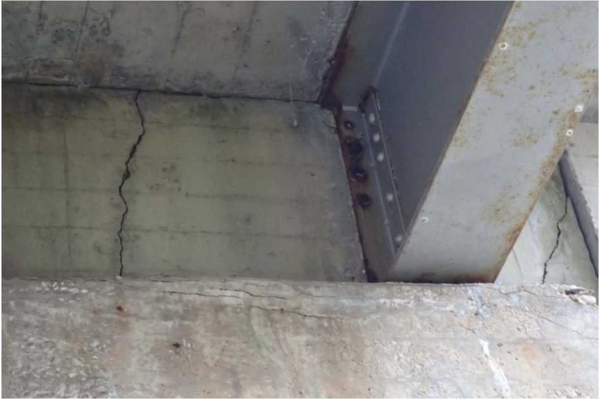
Typical view of beam 4 from upstream at abutment 2. Notice there is only minor rust/corrosion at this time. Notice the moderate sized vertical crack in the adjacent backwall/diaphragm.
