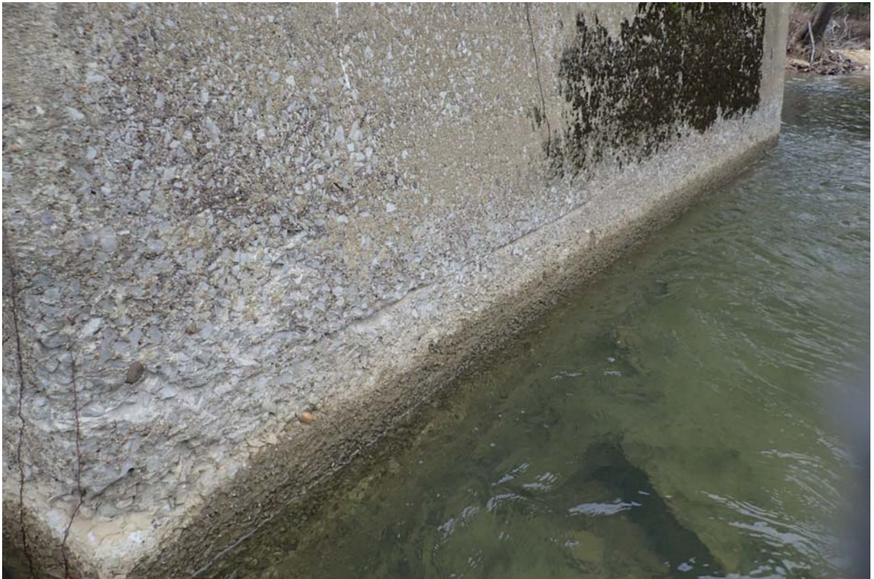
Moderate scaling along the flowline of abutment 1.
