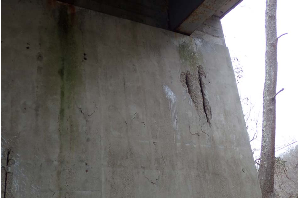
Moderate spalling with exposed steel in abutment 1 below the upstream beam.
