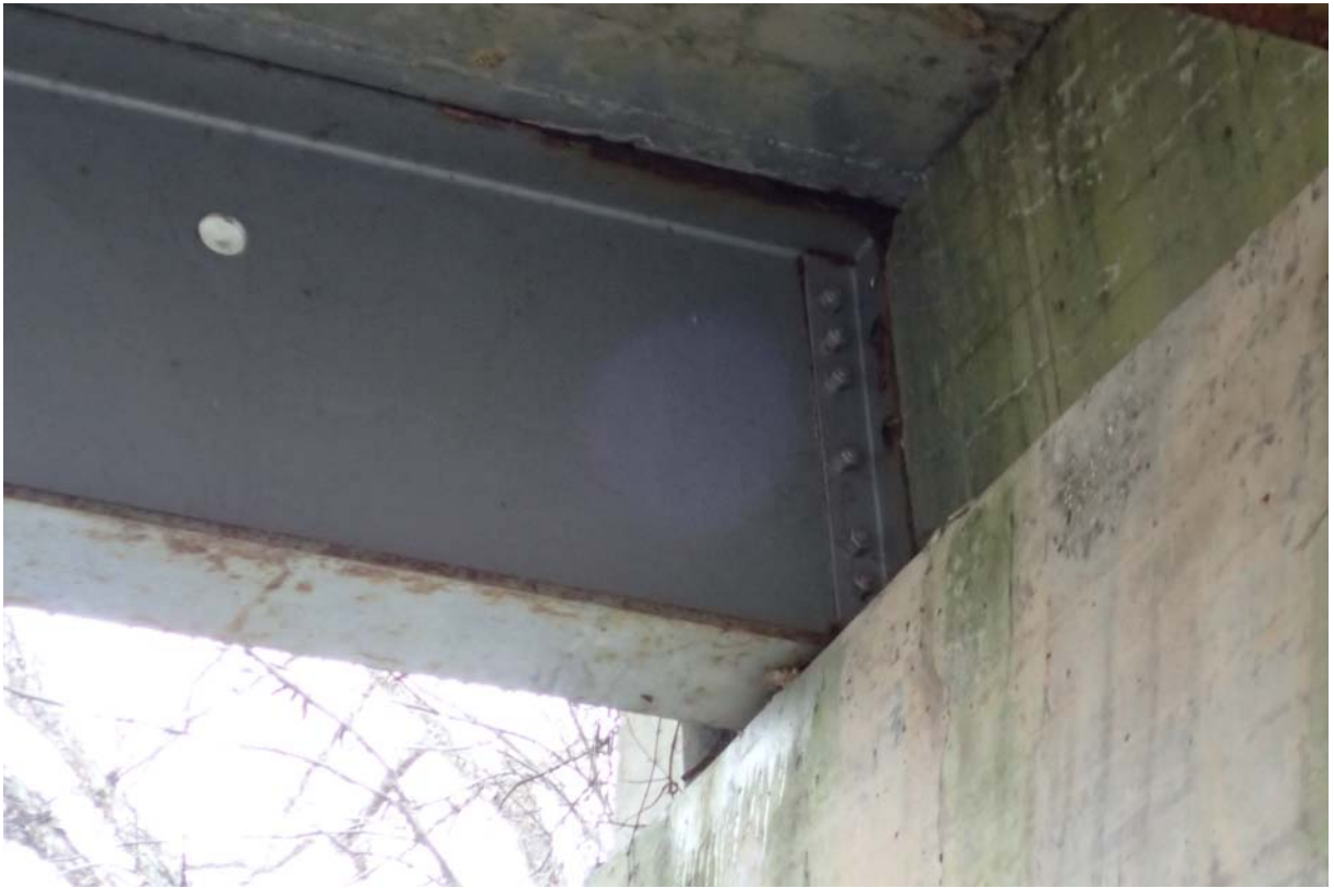
Typical view of beam 4 from upstream at abutment 1. Notice the minor rust/corrosion of the flanges.
