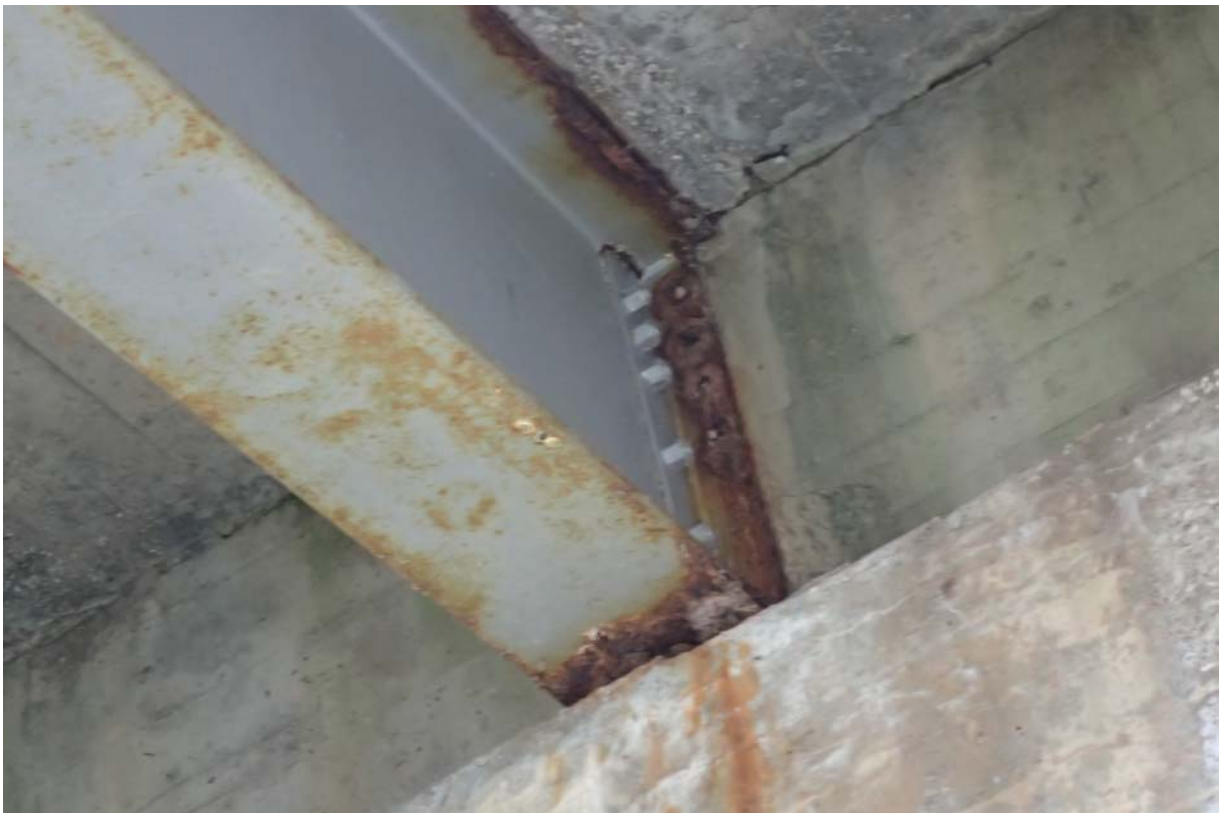
Typical view of beam 3 from upstream at abutment 2. Notice the moderate rust/corrosion of the flanges.
