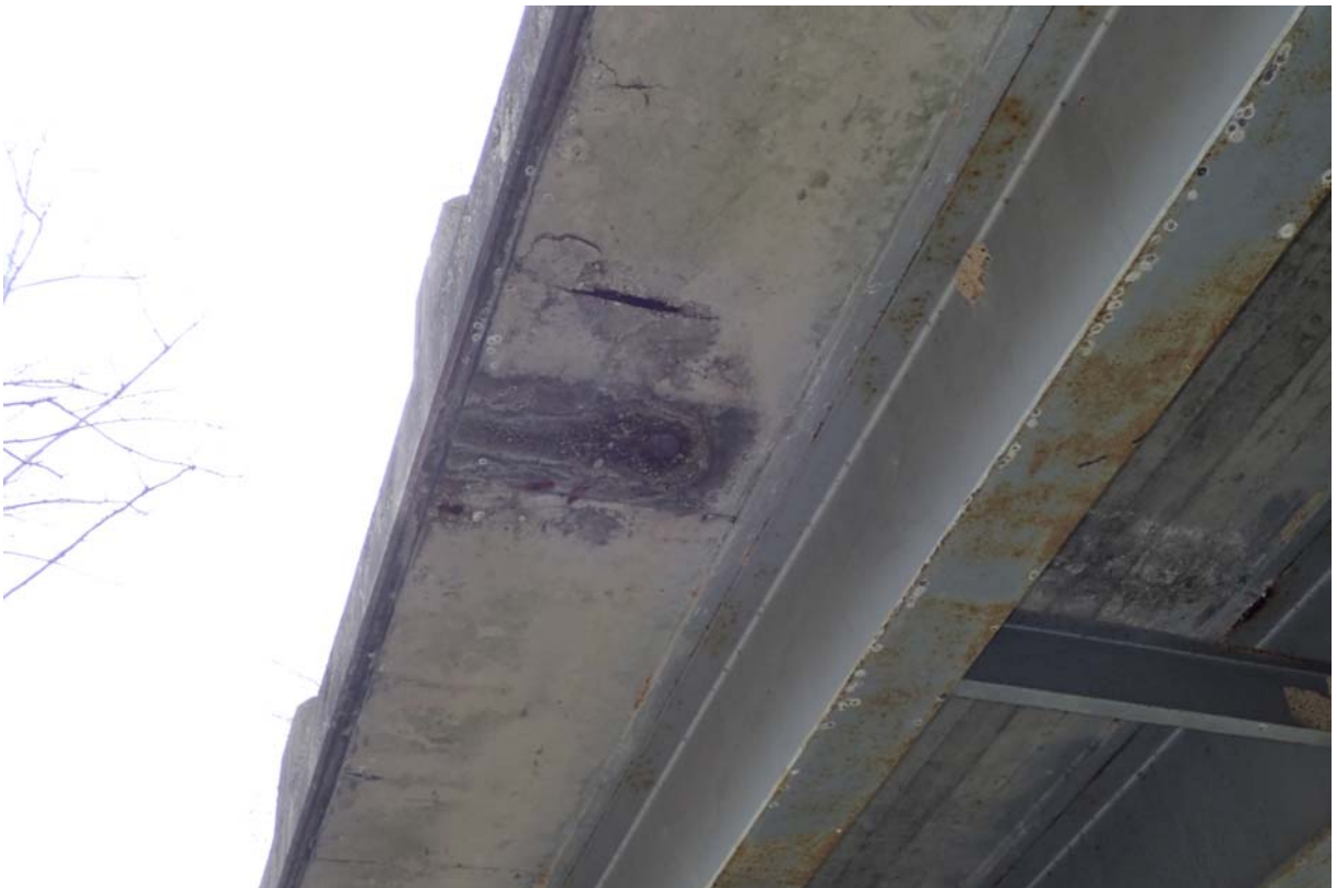
Spalling with exposed steel, delamination cracking, and discoloration in the upstream deck overhang.
