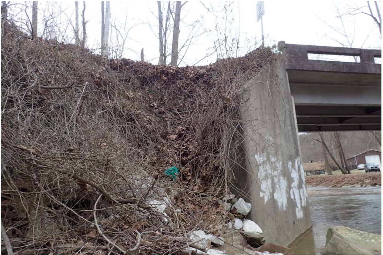
Heavy embankment erosion adjacent to abutment 2.
