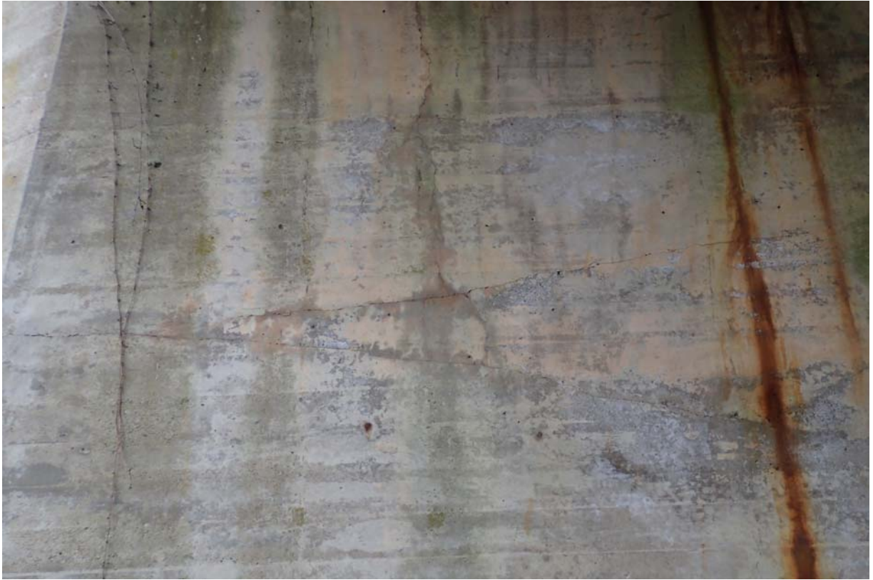
Minor sized horizontal, diagonal, and vertical cracking in abutment 1 between beams 3 and 4 from upstream.
