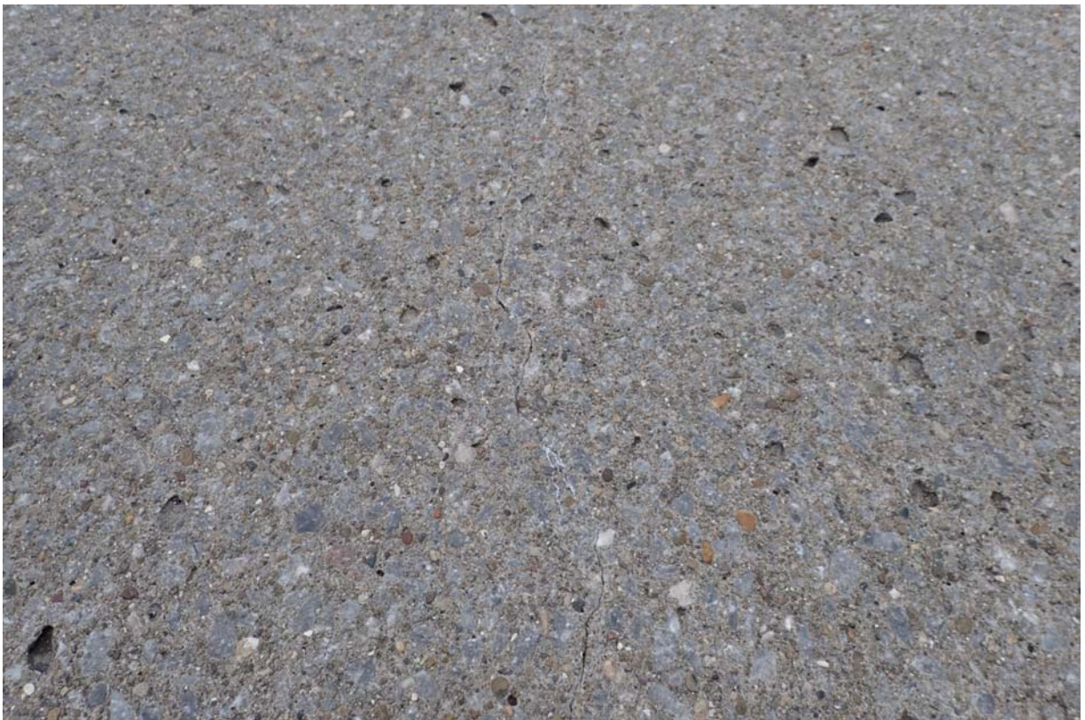
Minor sized transverse cracking in the wearing surface near mid-length.
