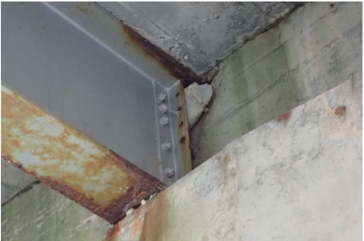
Typical view of beam 3 from upstream at abutment 1 (upstream face). Notice the moderate rust/corrosion of the web and flanges. Also notice the piece of concrete behind the vertical angle at the end of the beam.
