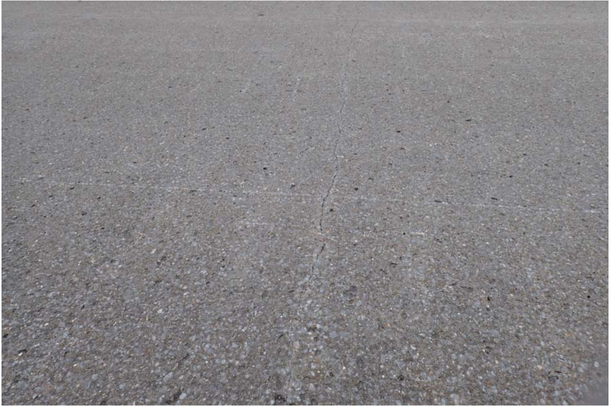
Minor sized transverse cracking in the wearing surface near abutment 1.
