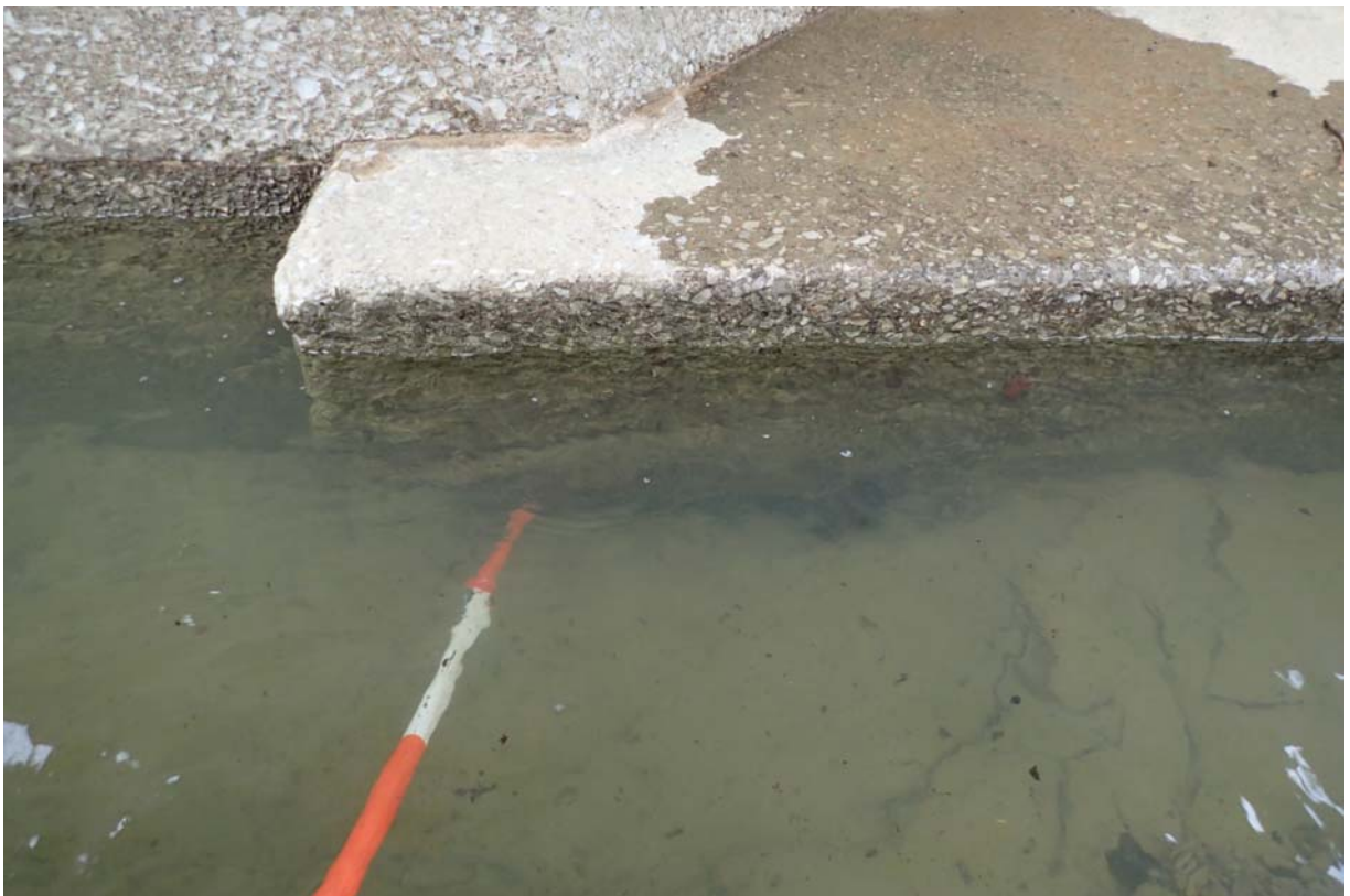
Up to 6" of horizontal undermining under the downstream portion of the newer footing of abutment 1. This extends for ~3' in length.
