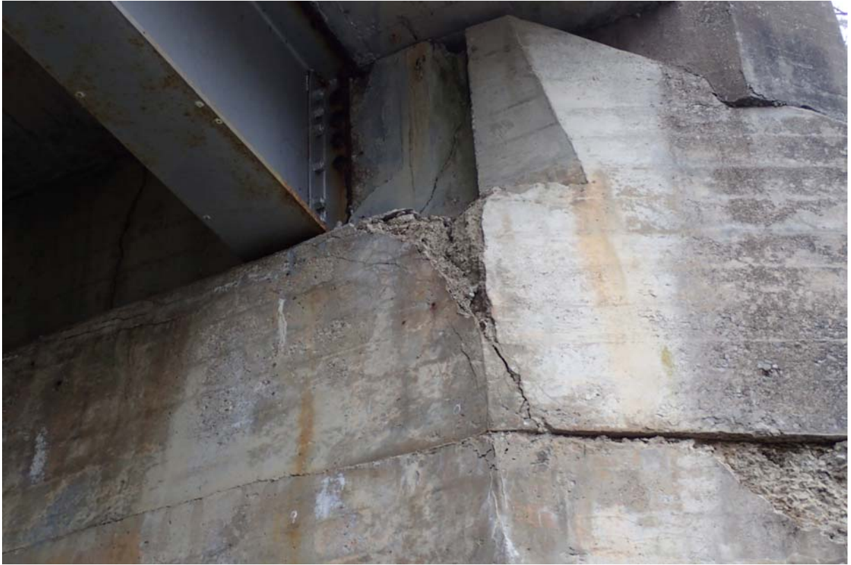
Moderate to heavy cracking/spalling in abutment 2 adjacent to the downstream exterior beam.
