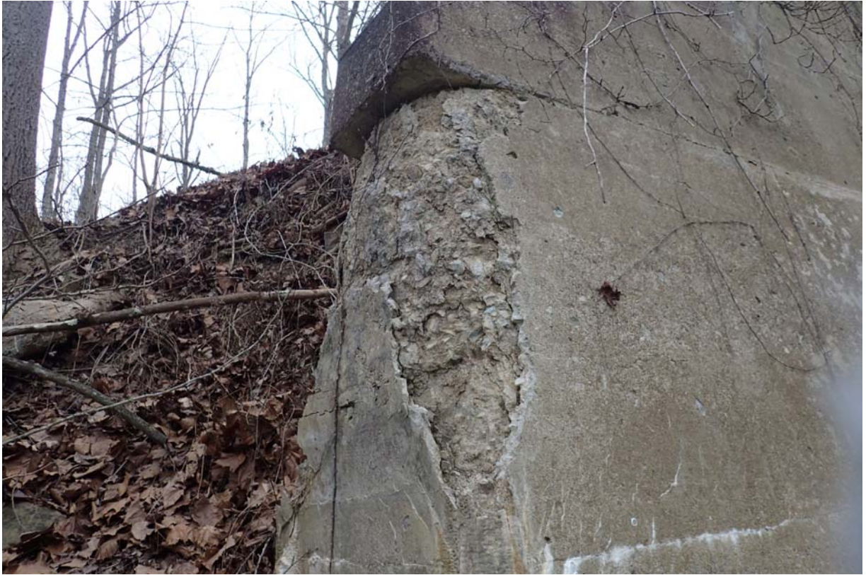
Moderate to heavy spalling at the downstream end of abutment 1s downstream wingwall.
