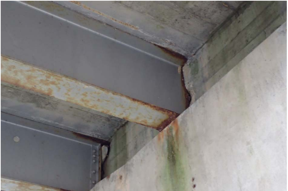
Typical view of beam 2 from upstream at abutment 1. Notice the moderate rust/corrosion of the web and flanges.
