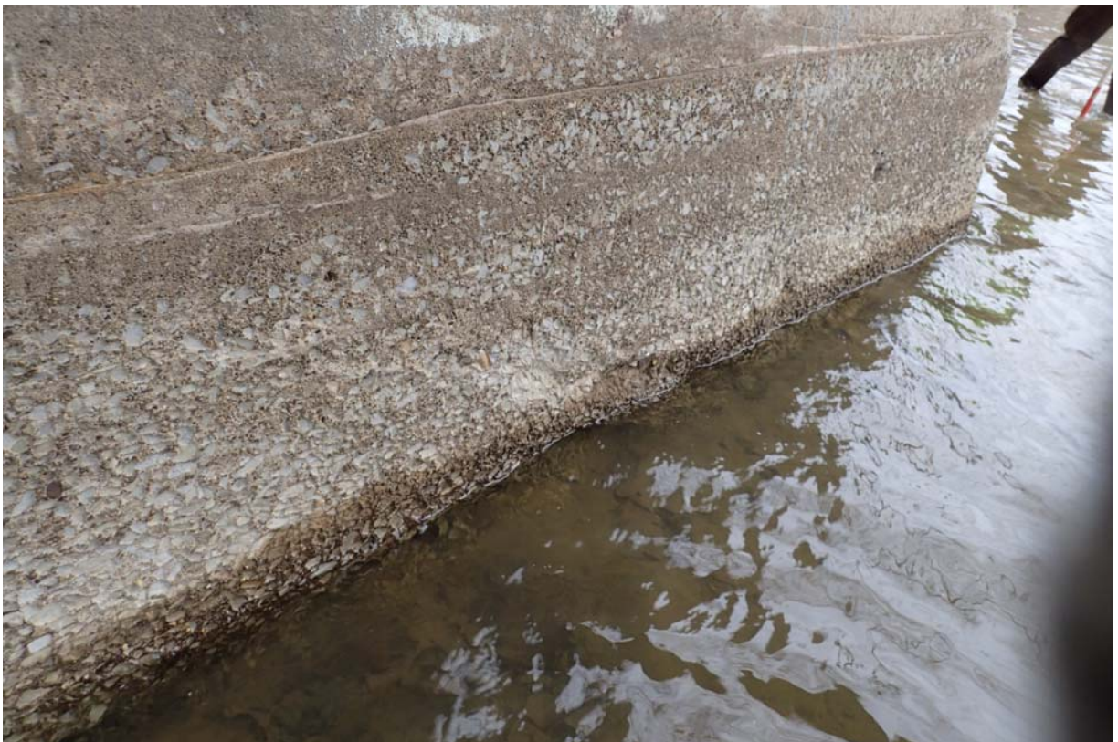
Moderate scaling along the flowline of abutment 2.
