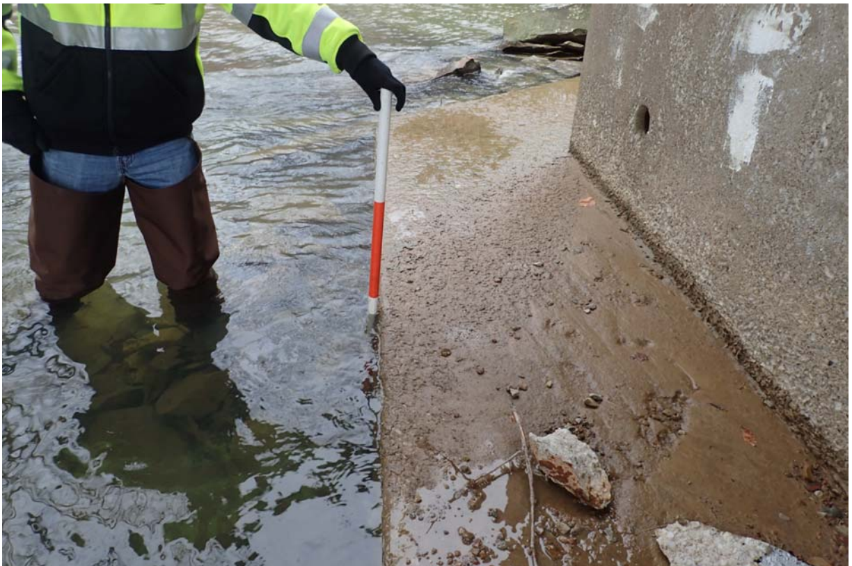
Abutment 2s footing is vertically exposed ~ 2' at the upstream end.
