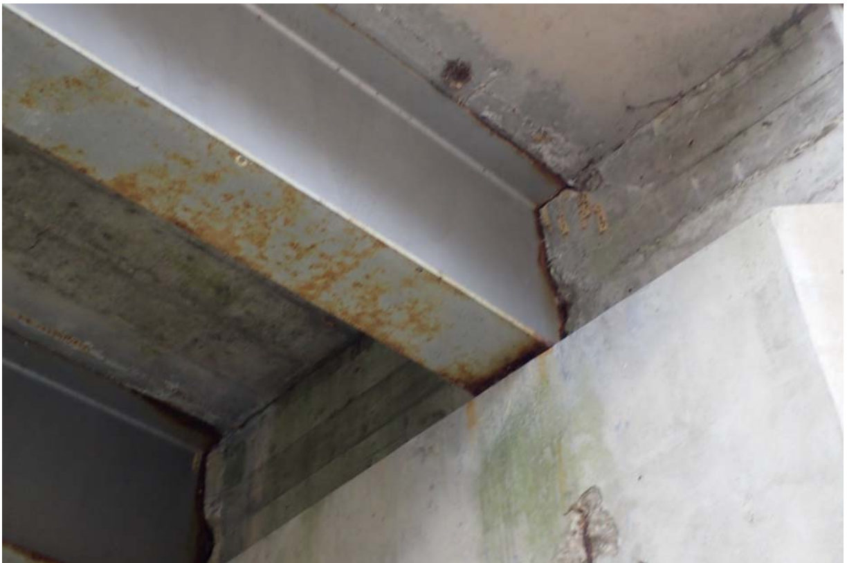
Typical view of the upstream beam at abutment 1. Notice the moderate rust/corrosion of the web and flanges.
