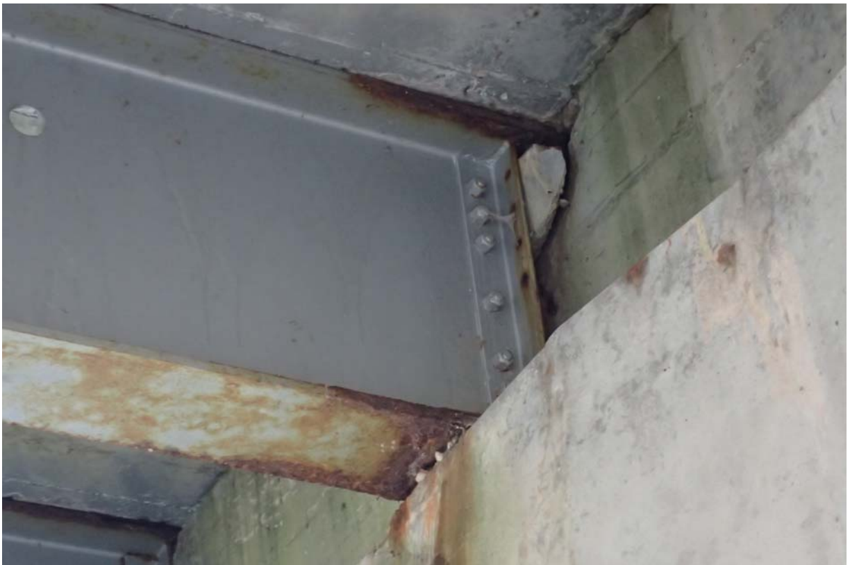
Typical view of beam 3 from upstream at abutment 1. Notice the moderate rust/corrosion of the web and flanges. Also notice the piece of concrete behind the vertical angle at the end of the beam.
