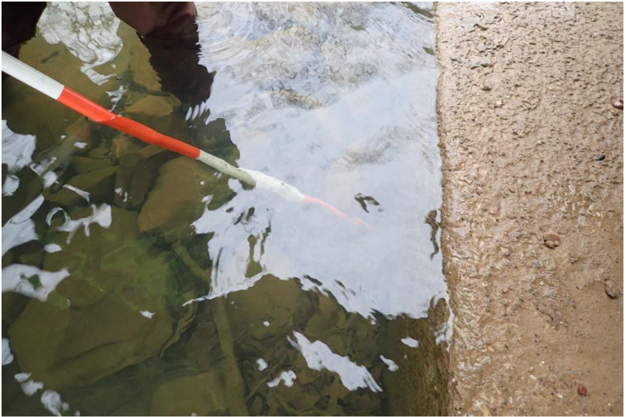
Approximately 2" of horizontal undermining along the upstream footing of abutment 2. This extends for ~ 3' in length.
