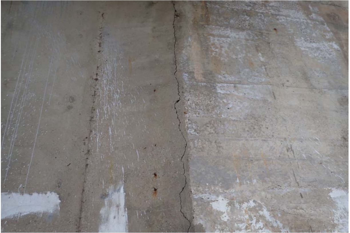
Minor sized vertical crack in abutment 2 near the old/new abutment interface.
