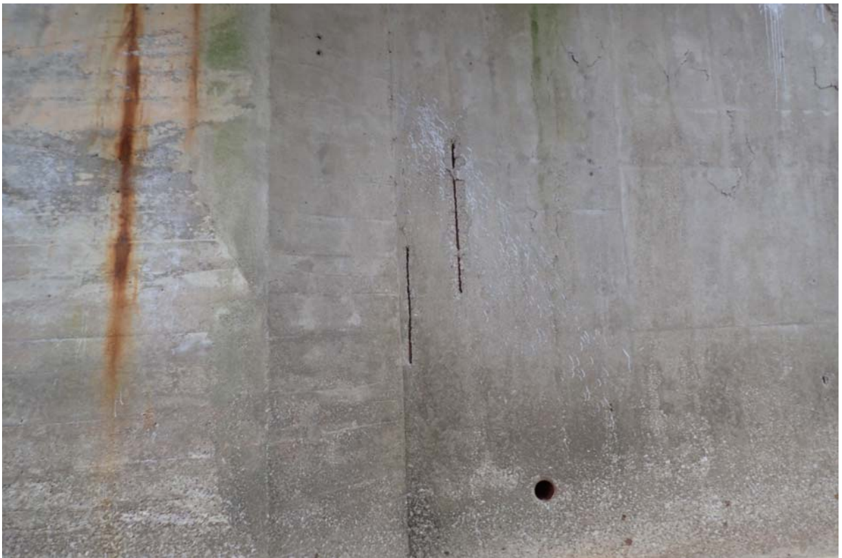
Moderate spalling with exposed steel in abutment 1 near the centerline of the abutment.
