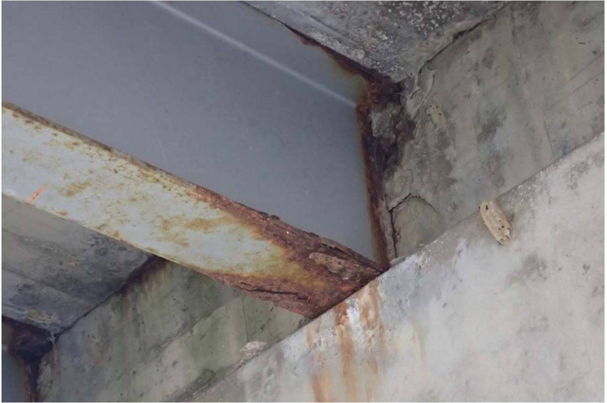
Typical view of beam 2 from upstream at abutment 2. Notice the moderate rust/corrosion of the web and flanges.
