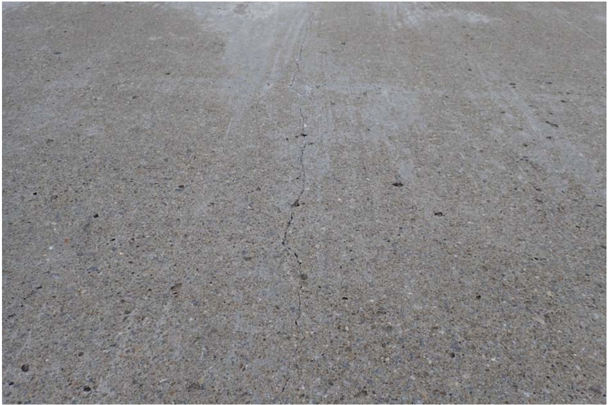
Minor sized transverse cracking in the wearing surface near abutment 2.
