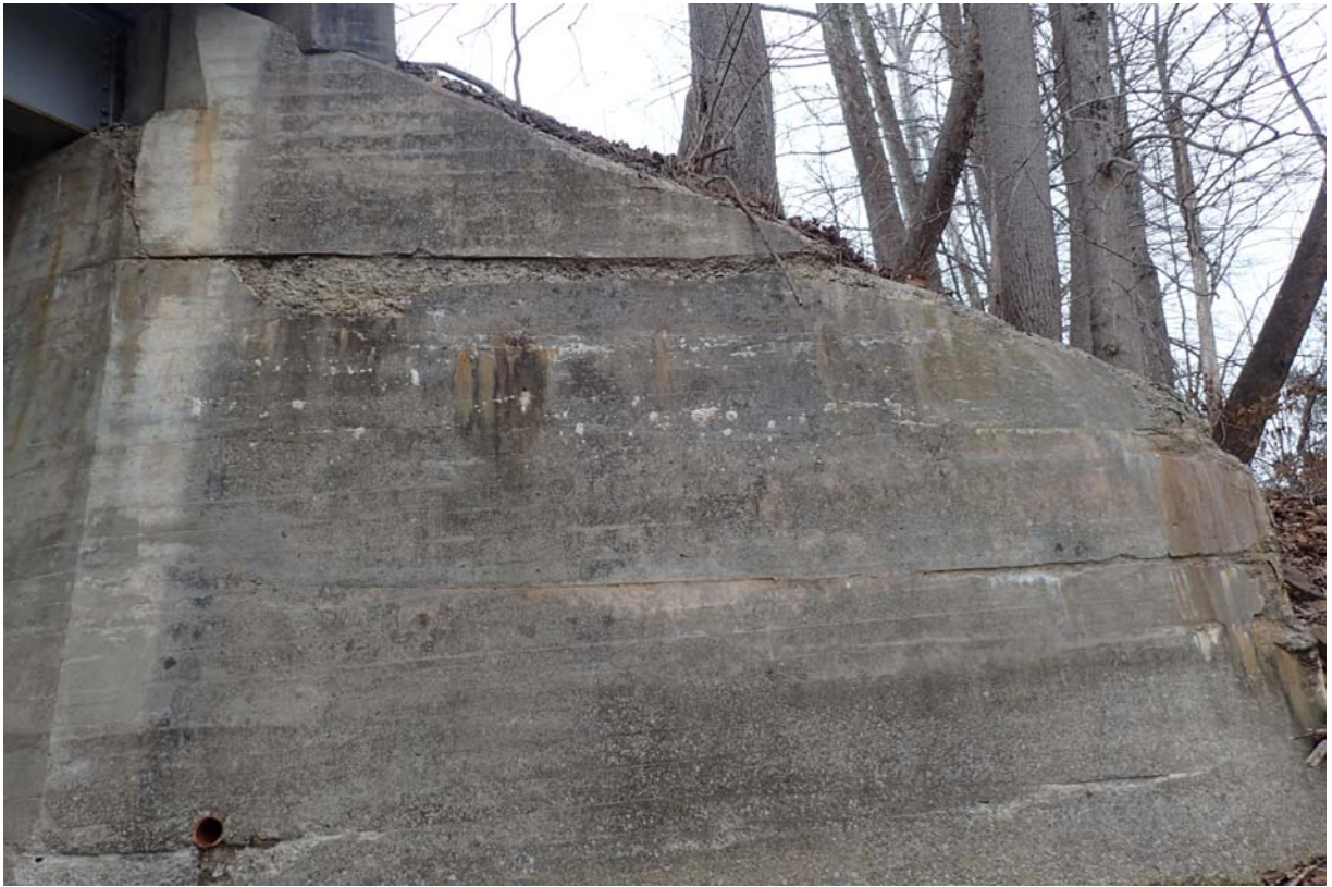
Spalling near and along the top of abutment 2s downstream wingwall.
