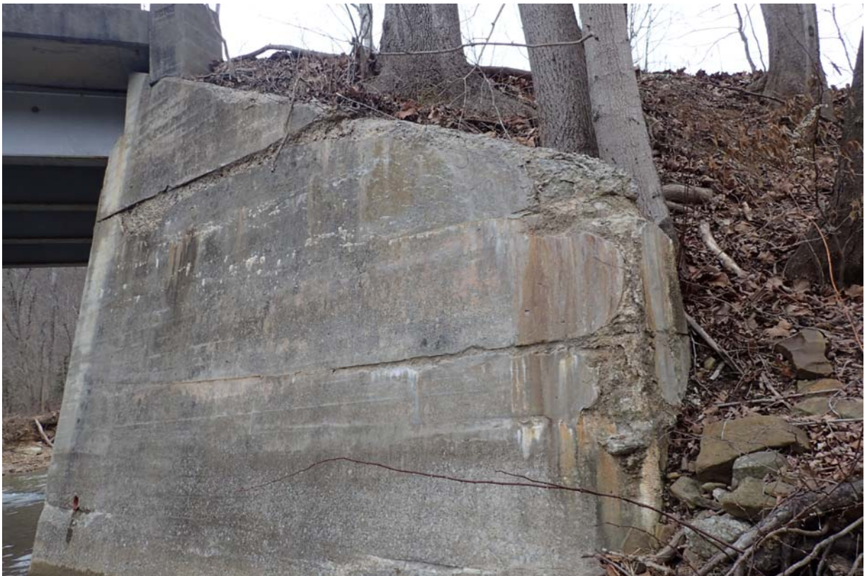
Spalling along the top and at the end of abutment 2s downstream wingwall.
