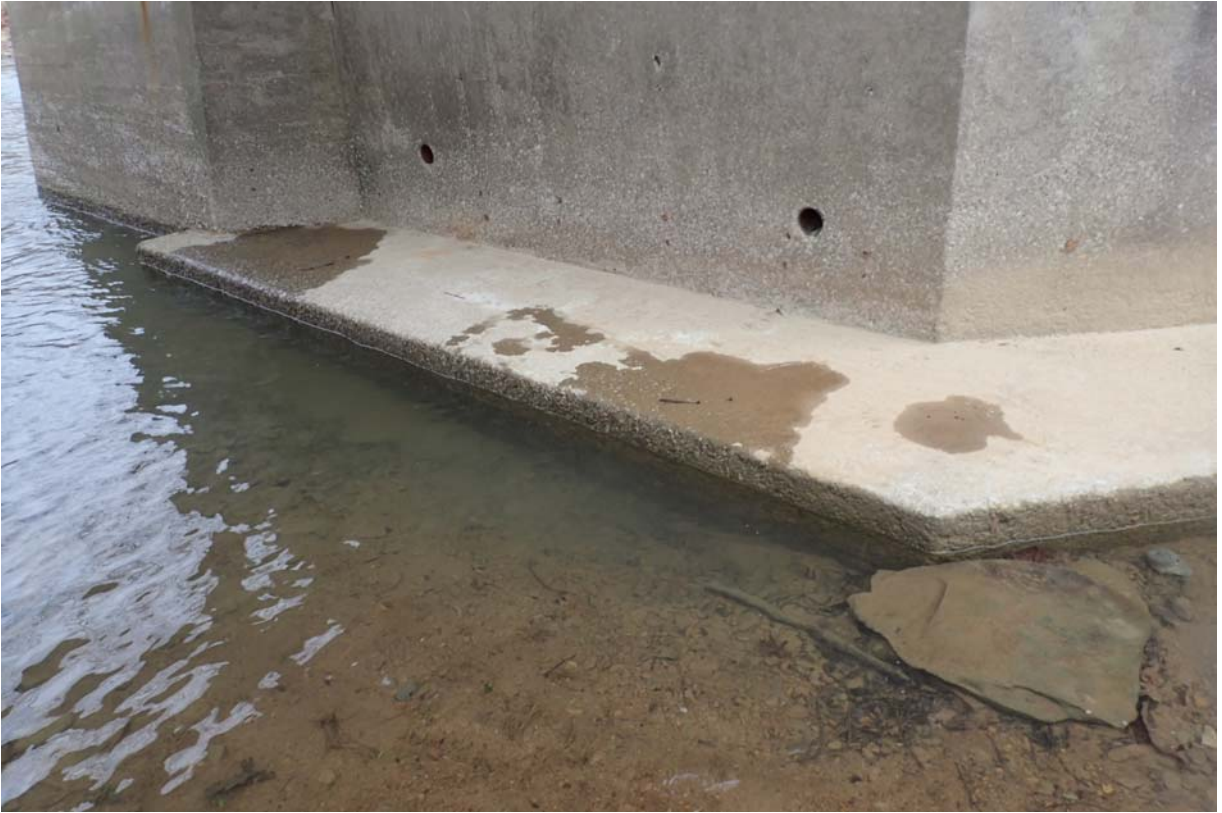
Exposed upstream footing of abutment 1.
