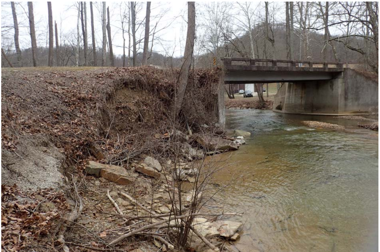
Heavy embankment erosion just upstream of abutment 2.
